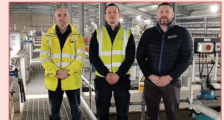
Energy efficiency LED lighting at Drummaroad water treatment works, County Down.
