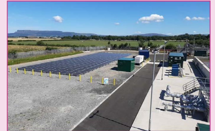
Solar powered battery energy system at Ballykelly wastewater treatment works, County Derry/Londonderry.
